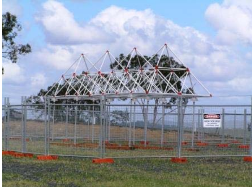
Figure 1: ATLANT system installed at Paradise Dam, Queensland, 2008
